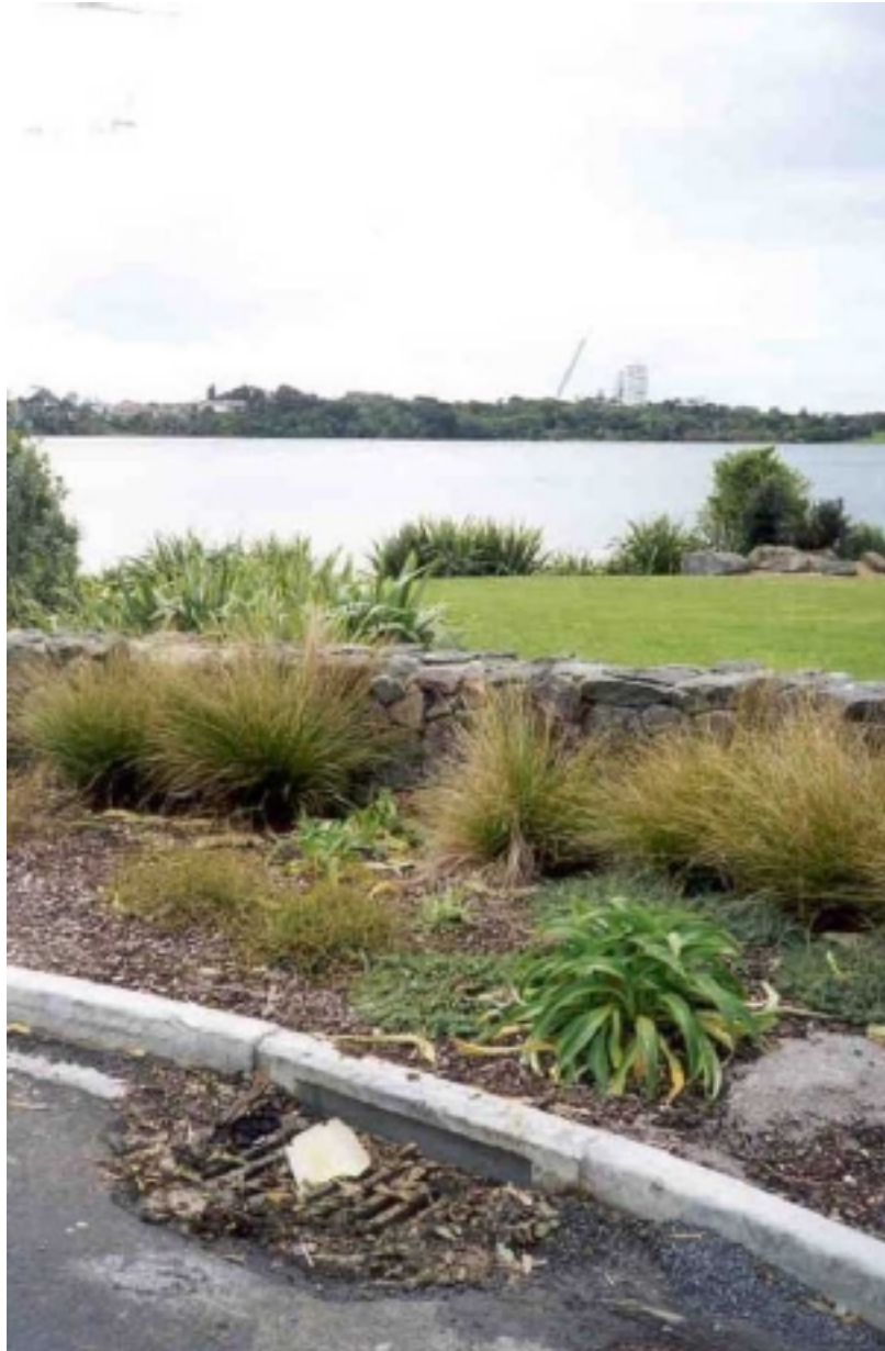
PHOTO 2: Shea Terrace catchpit showing deposition of organics, litter and metal View from the bottom of Shea Terrace, looking northeast towards Lake Pupuke
