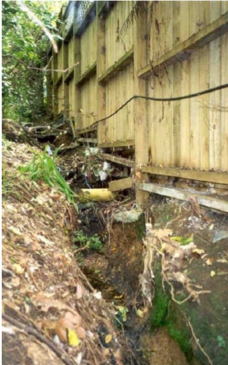
Photo 4: Scouring as a result of stormwater discharging from a pipe approx. 10m back upstream
