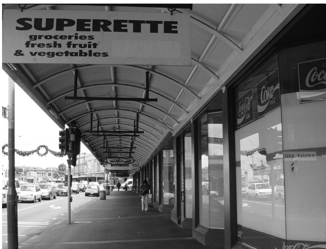
In the past verandahs were supported on posts (often decorated) at the kerbside, creating an arcade-like space - perforated screen between the road and the footpath
