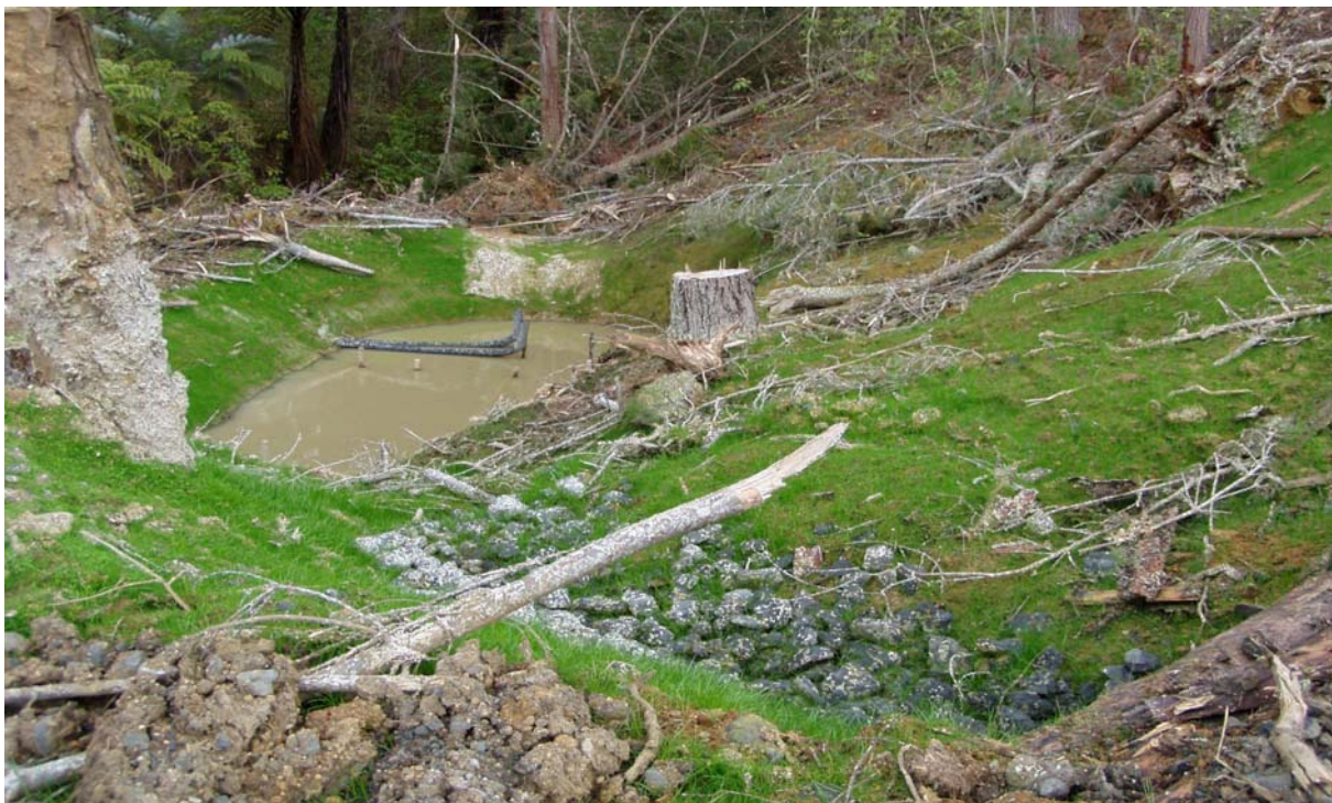
Photo 7.6 An example of a Decanting Earth Bund. The DEB was installed with a decanted outlet as it was treating a maximum catchment area of 3,000m 2 .
