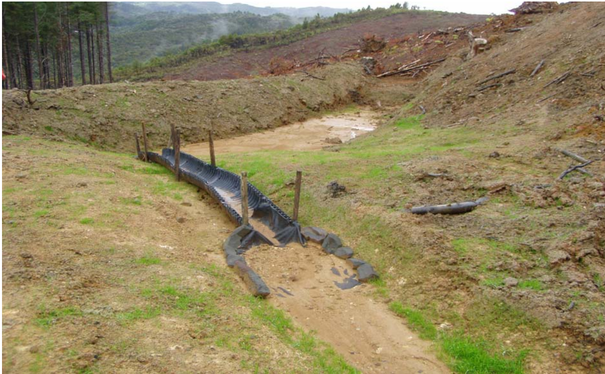
Photo 7.5 An example of an earth bund installed downslope of road works. This earth bund was constructed for a contributing catchment of less than 1000m 2 and therefore did not require a decanting outlet. Note optional use of flume to convey sediment-laden flows.
