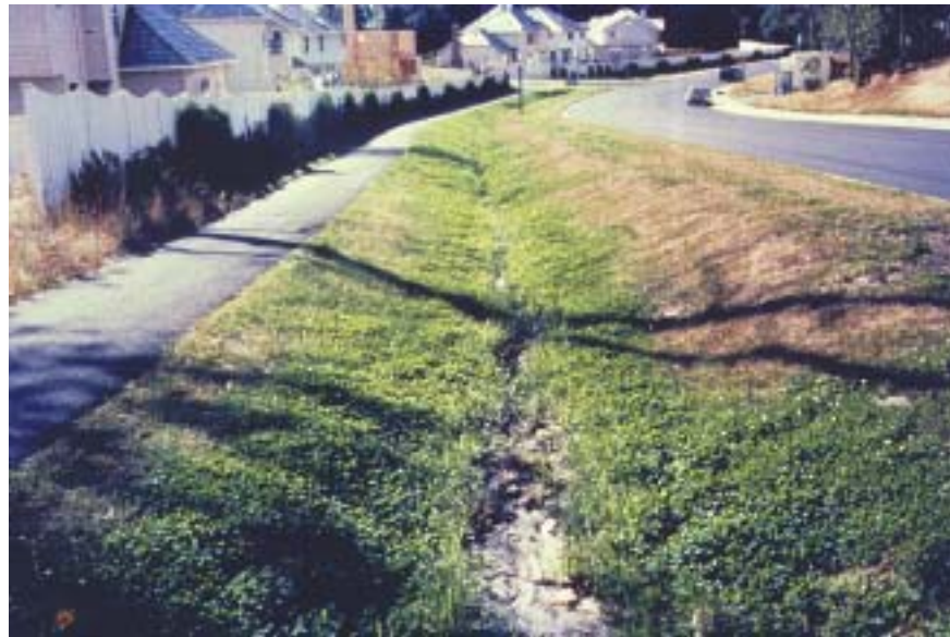
Plate 9-6: Swale needing maintenance due to high sediment loads
